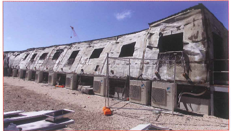
Canteen facilities at Nauru Detention Centre damaged by rioting in 2013
